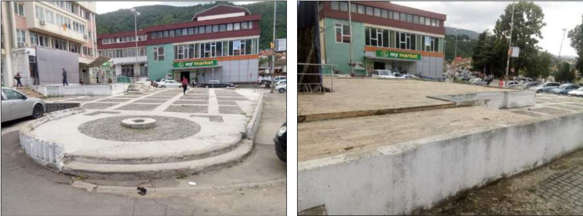
Fig. 3 - Current state of the stage on the square (obsolete, damaged and completely dysfunctional)
